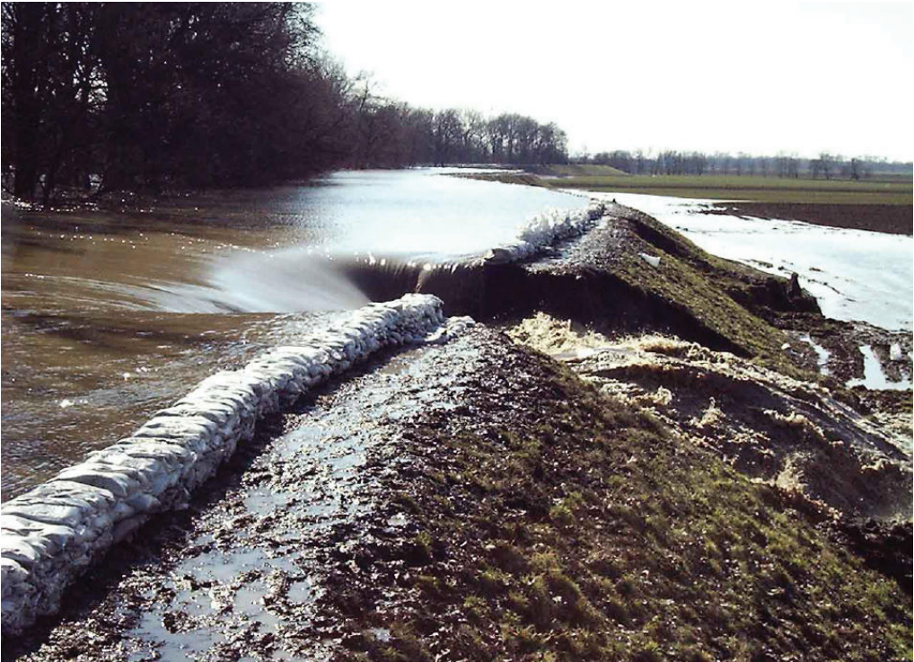
PICTURE 1 ♦ Dam break in Tarpa. (Photo: www.tarpa.eu )
